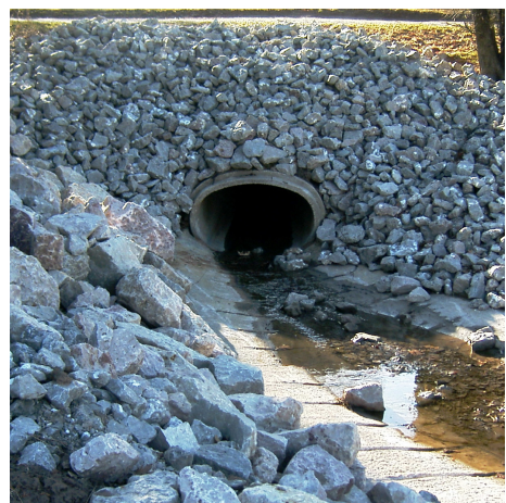
Photo 3.7.3: 29"x54" Golf Course Outfall
