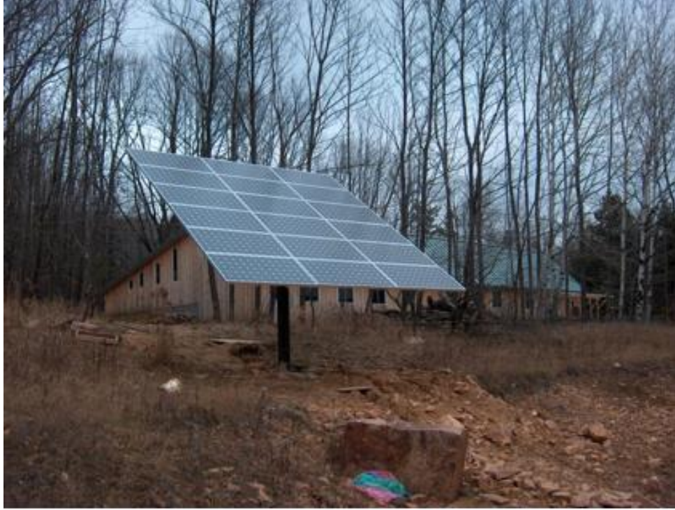
Example of a 3.2 kW pole mounted, fixed array that is seasonally adjustable.
