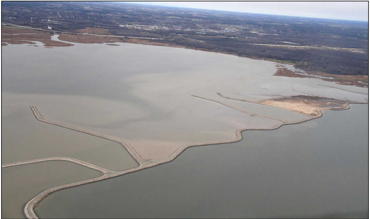
Photograph of the Cat Island Wave Barrier facing southwest towards the mouth of Duck Creek. Photograph taken by Erin Giese on 2 December 2016.
